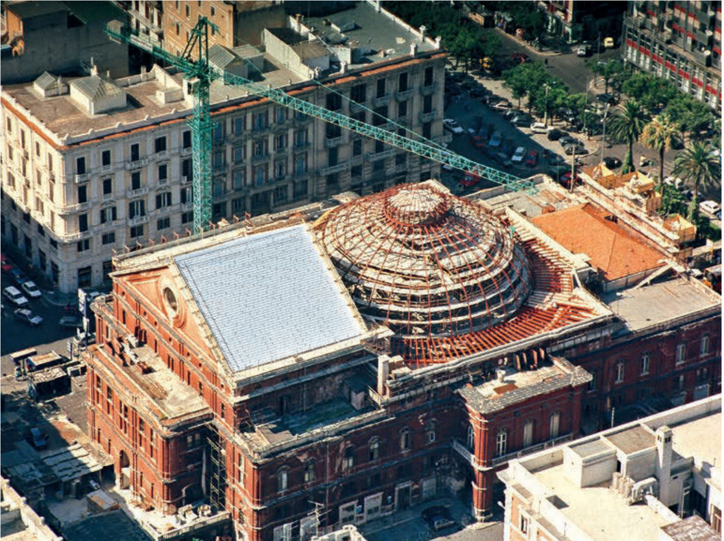
Bari - Isotec Insulation of the roofing during the works for the rebuilding of Teatro Petruzzelli.
