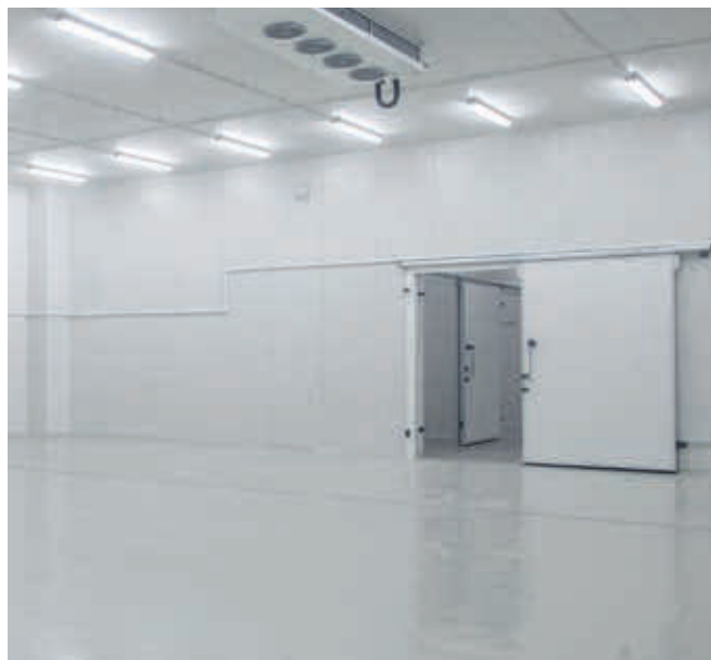
Cold storage rooms
